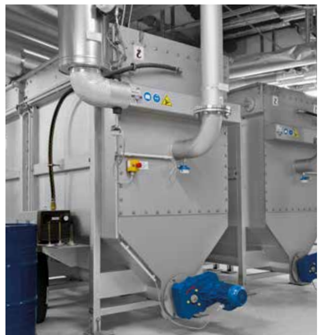
Municipal wastewater; 2x RoWin BG8; therm. extraction capacity 560 kW heating/1000 kW cooling.
