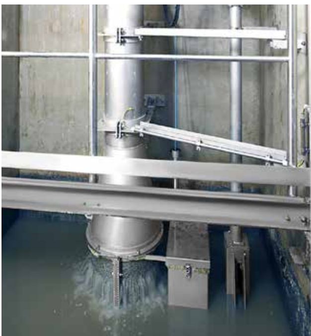
Wastewater pre-screening in the intake structure with a HUBER Pumping Stations Screen ROTAMAT® RoK4.
