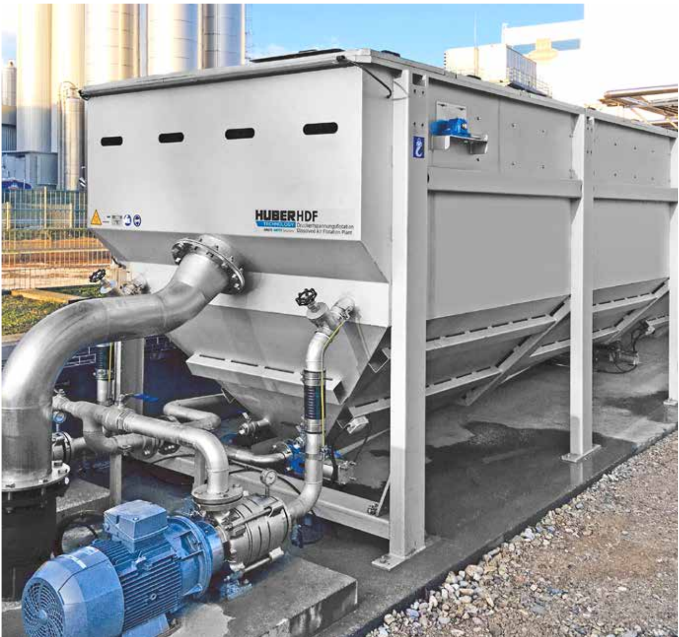
HUBER Dissolved Air Flotation Plant HDF S installed for activated sludge separation.
