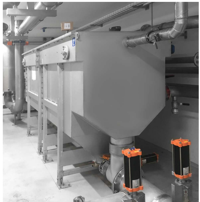
HUBER Heat Exchanger RoWin for heat recovery and wastewater cooling – energy optimisation and compliance with temperature limits.
