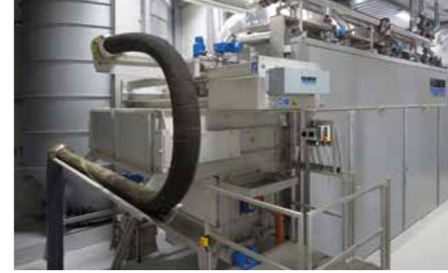
Sludge feeding with HUBER extruder unit.
