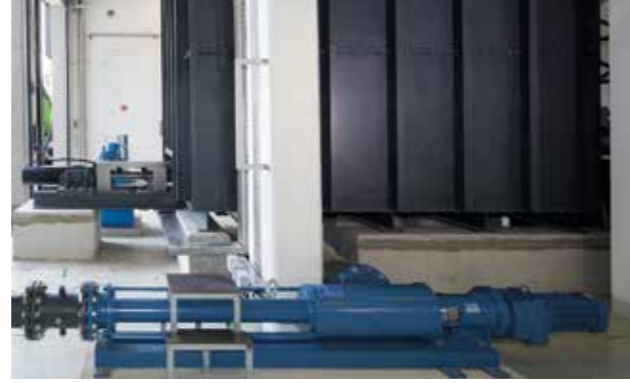
Sludge bunker and pump.
