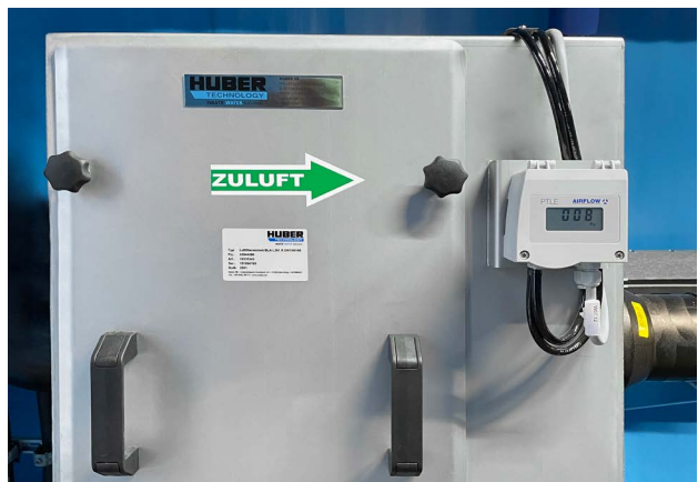
HUBER Aeration/Deaeration Plant L361.
