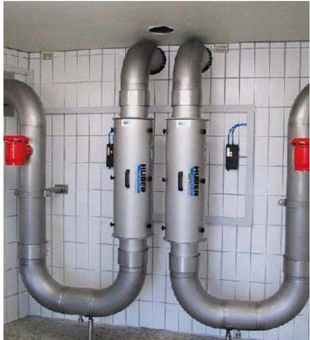
HUBER Aeration/Deaeration Plant L252.
