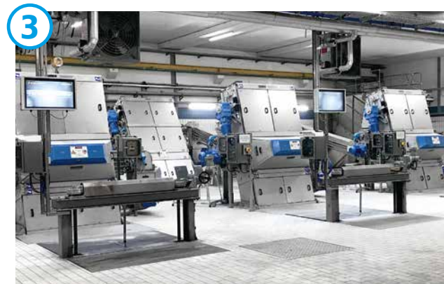
3 Sewage treatment plant Vohburg Sewage treatment plant Nuremberg
