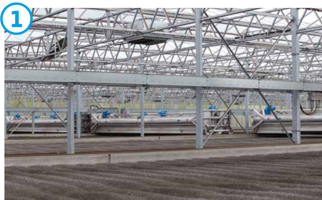
1 Sewage treatment plant Bayreuth
