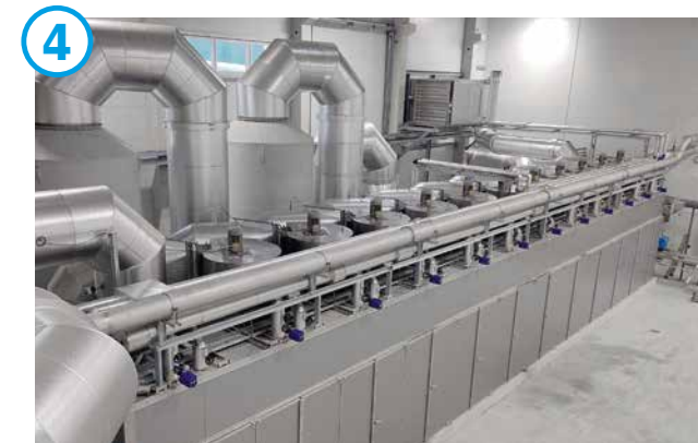
4 Emter GmbH in Altenstadt + Sewage treatment plant Penzing
