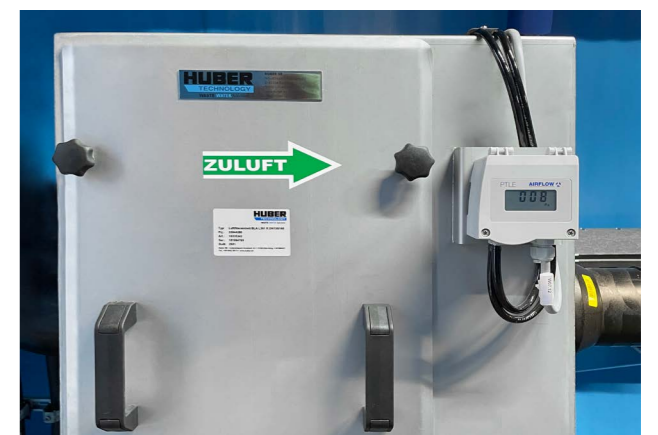
HUBER Aeration/Deaeration Plant L361.
