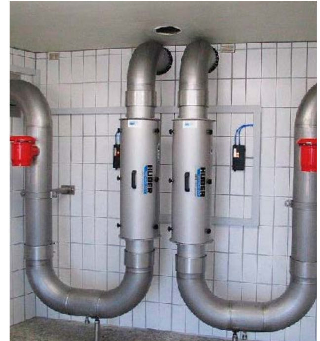
HUBER Aeration/Deaeration Plant L252.
